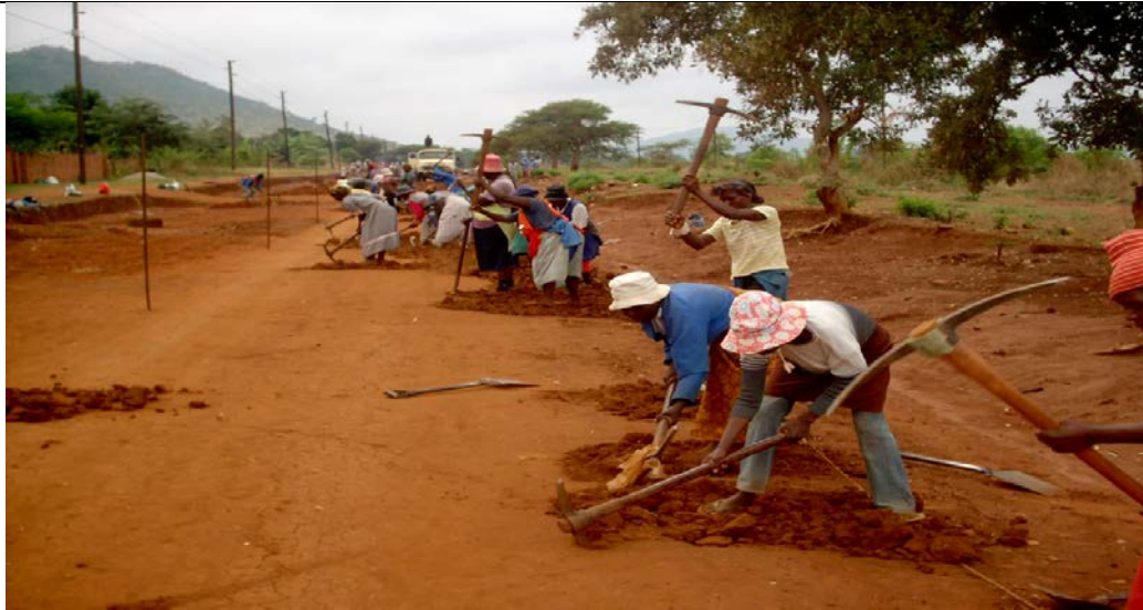
Picture 5: Labour intensive methods create jobs and ensure skills transfer to communities
